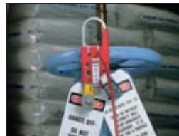
Lockout gate valves
